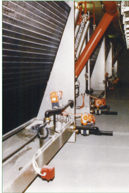
Figure 3: Hybrid coolers installed in a building
