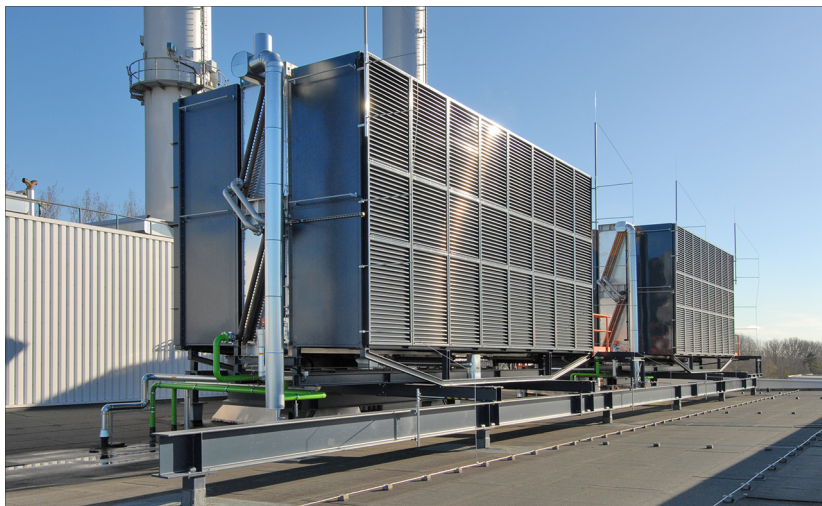
Figure 5. Air intake with hybrid combustion air conditioning and three-stage air filtration
